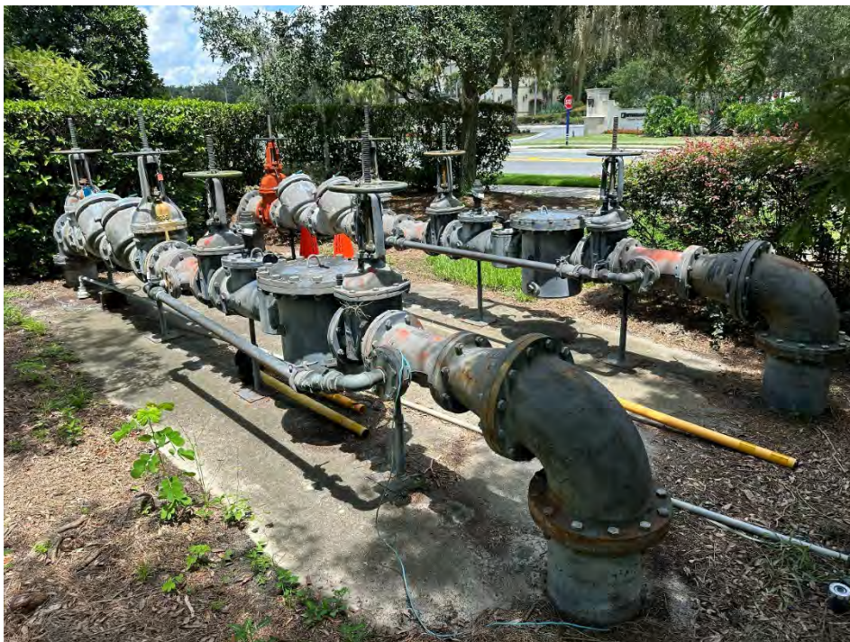
PHOTO 60 Backflow preventer assembly- paint coat fading
