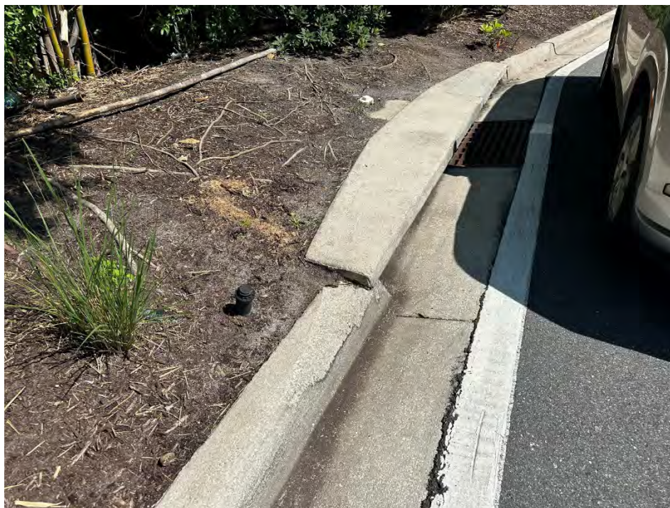
PHOTO 3 Concrete curb- broken/cracking near inlet
