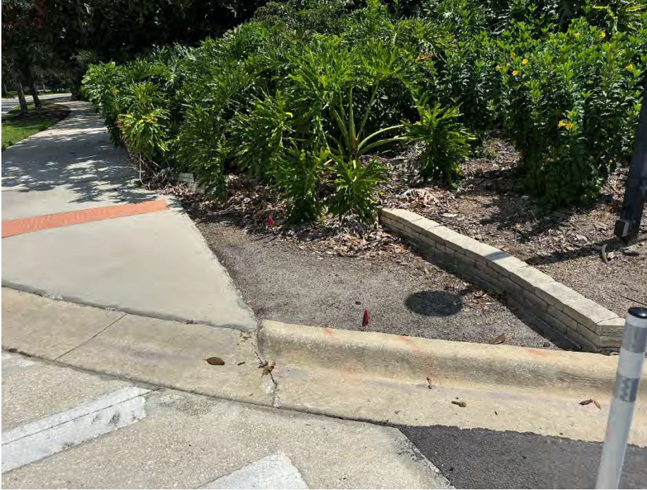
PHOTO 41 Brick wall- damaged/displaced
