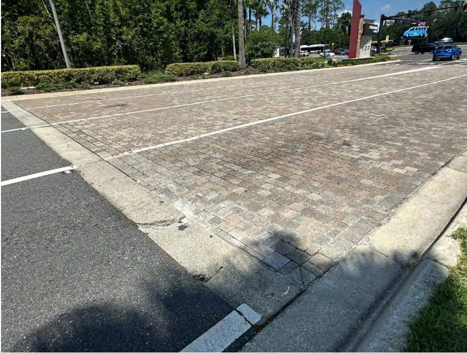
PHOTO 17 Brick paver- uneven, Concrete curb- broken/cracking
