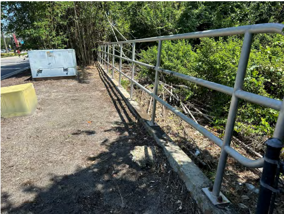
PHOTO 18 Metal railing – shifted/tilted
