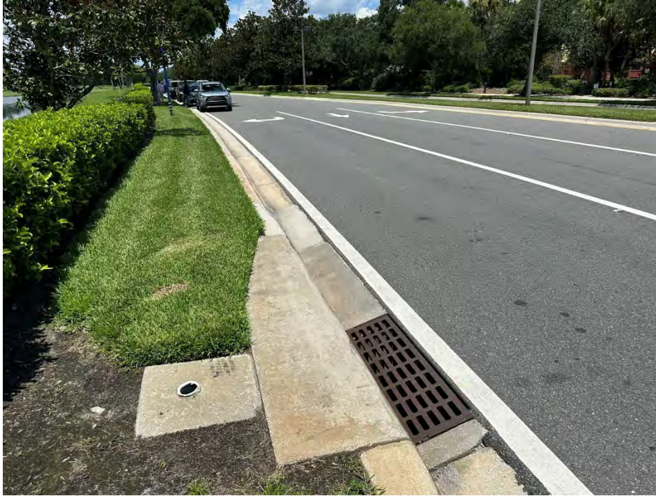
PHOTO 63 Underdrain cleanout- cap broken
