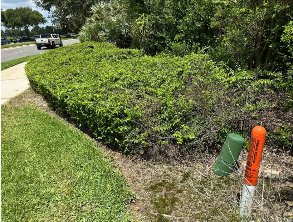
PHOTO 53 Communication covering- over-turned
