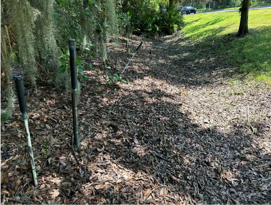
PHOTO 9 Lawn sprinklers- multiple are tilted and possibly no longer functional
