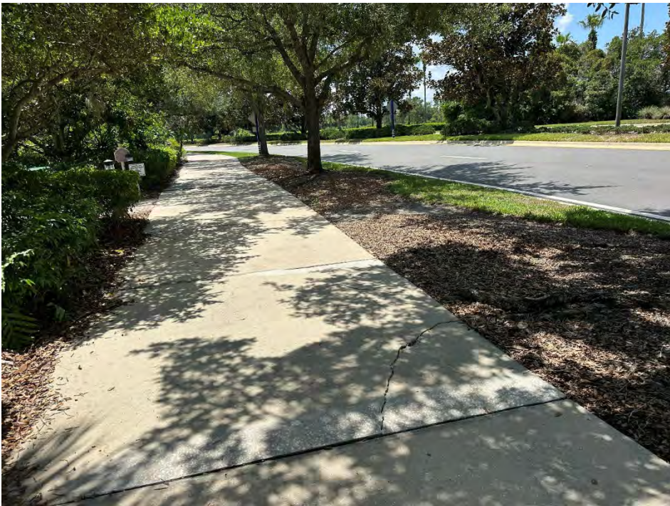
PHOTO 46 Sidewalk- broken/cracking, uneven at joints
