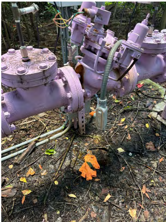
PHOTO 66 Irrigation backflow preventer assembly- leak observed
