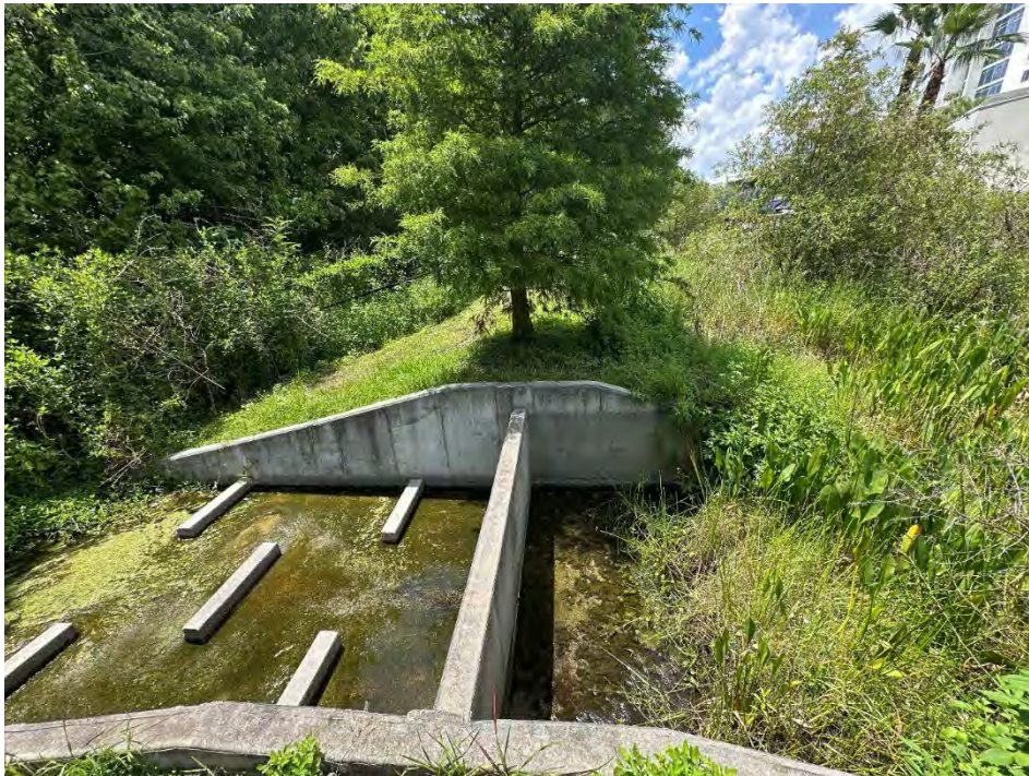
PHOTO 82 Concrete weir- excess vegetation growth
