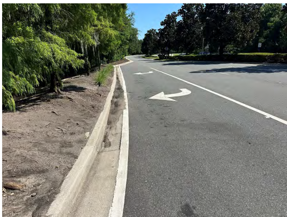
PHOTO 2 Concrete curb- sediment build up along gutter
