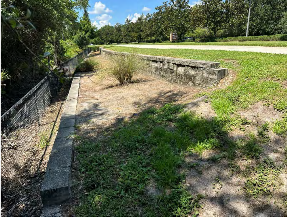
PHOTO 29 Irrigation lines- exposed
