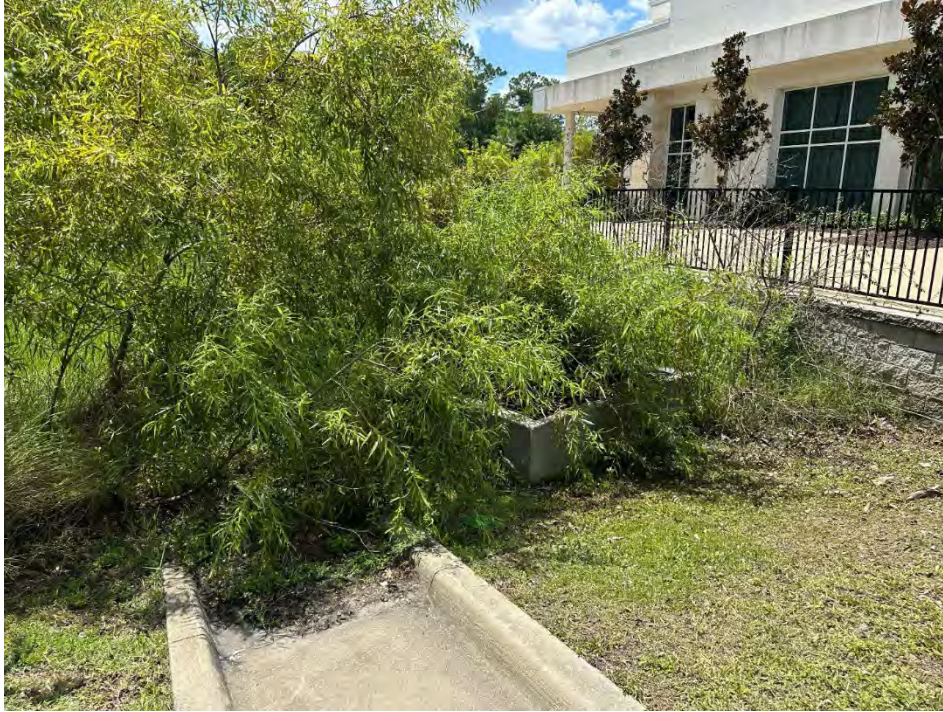
PHOTO 81 Control structure/flume- excess vegetation growth
