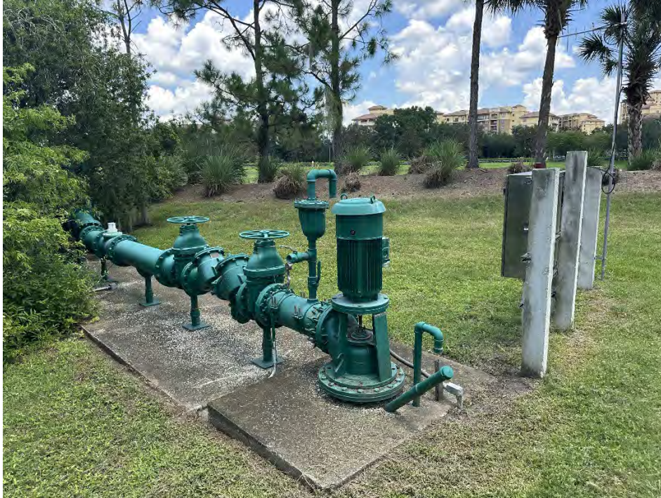
PHOTO 69 Irrigation pond backup well and manifold
