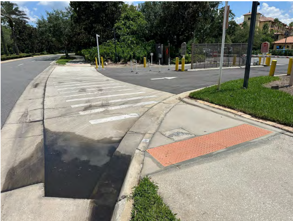
PHOTO 42 Concrete curb- broken/cracking, uneven at joints, holding water
