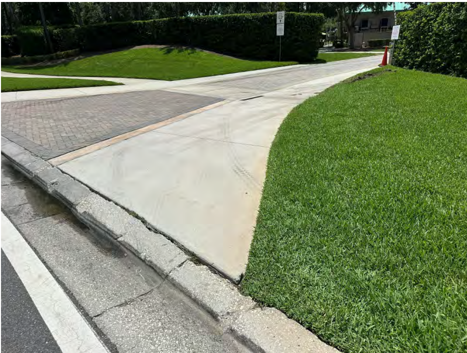
PHOTO 62 Concrete curb- broken/cracking
