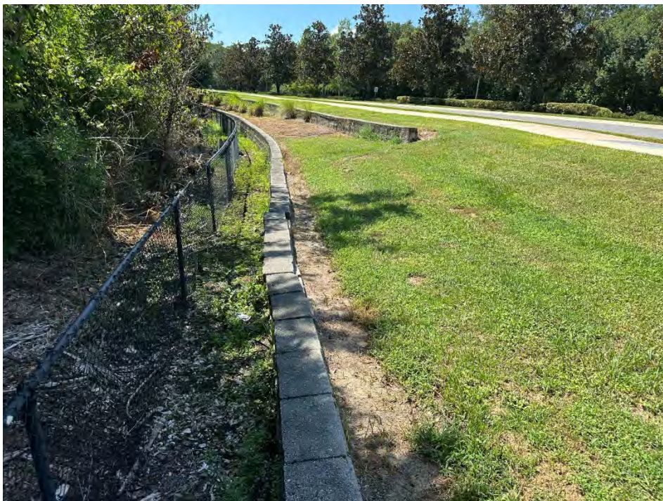
PHOTO 20 Retaining wall- blocks shifted/tilted
