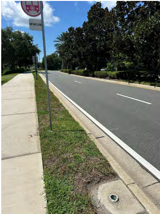
PHOTO 36 Underdrain cleanout- cap broken
