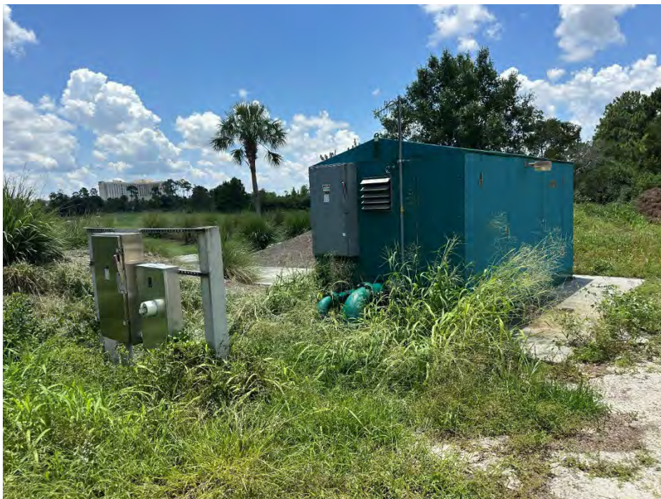
PHOTO 68 Pump house/electrical panel- excess vegetation growth impeding access
