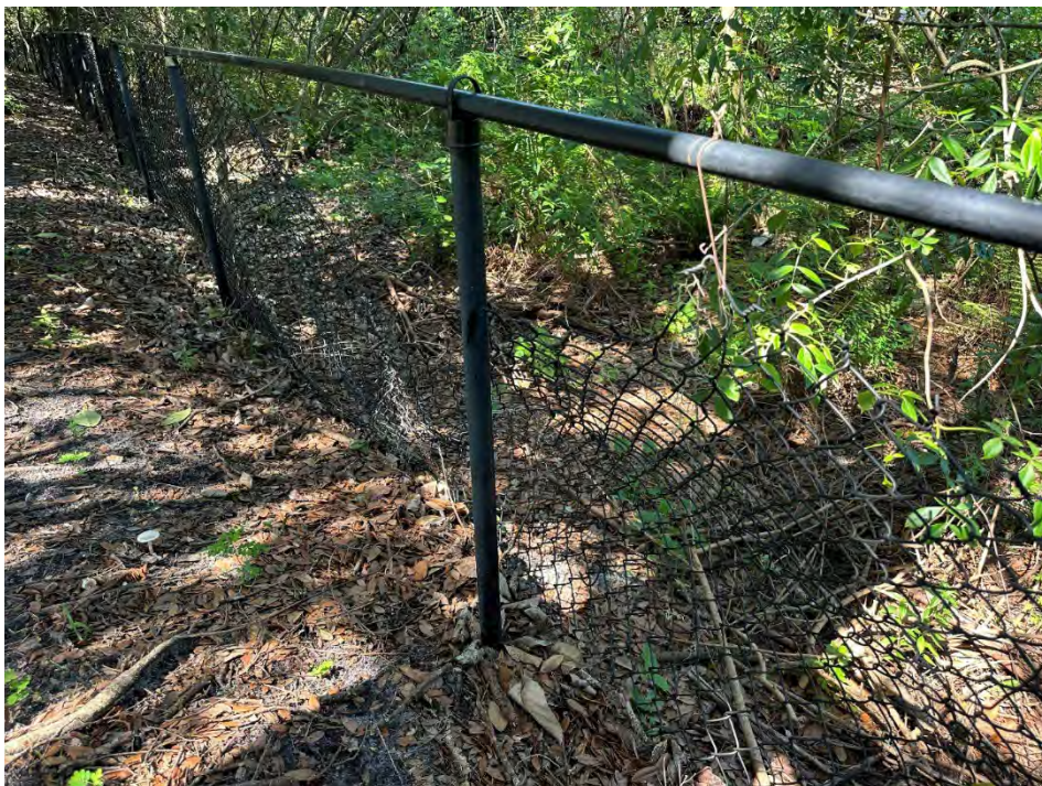
PHOTO 6 Chain link fence- several sections damaged and no longer intact/functional
