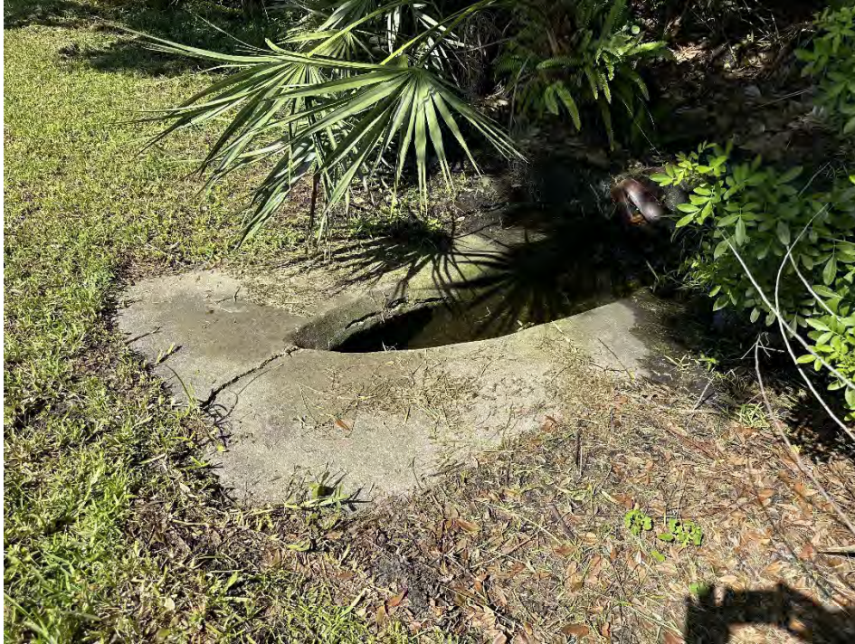
PHOTO 5 Mitered end section- with cracks in concrete
