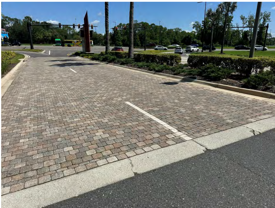
PHOTO 16 Concrete curb- broken/cracking
