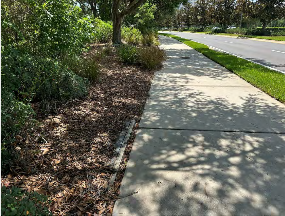
PHOTO 49 Electrical junction box- excess debris covering
