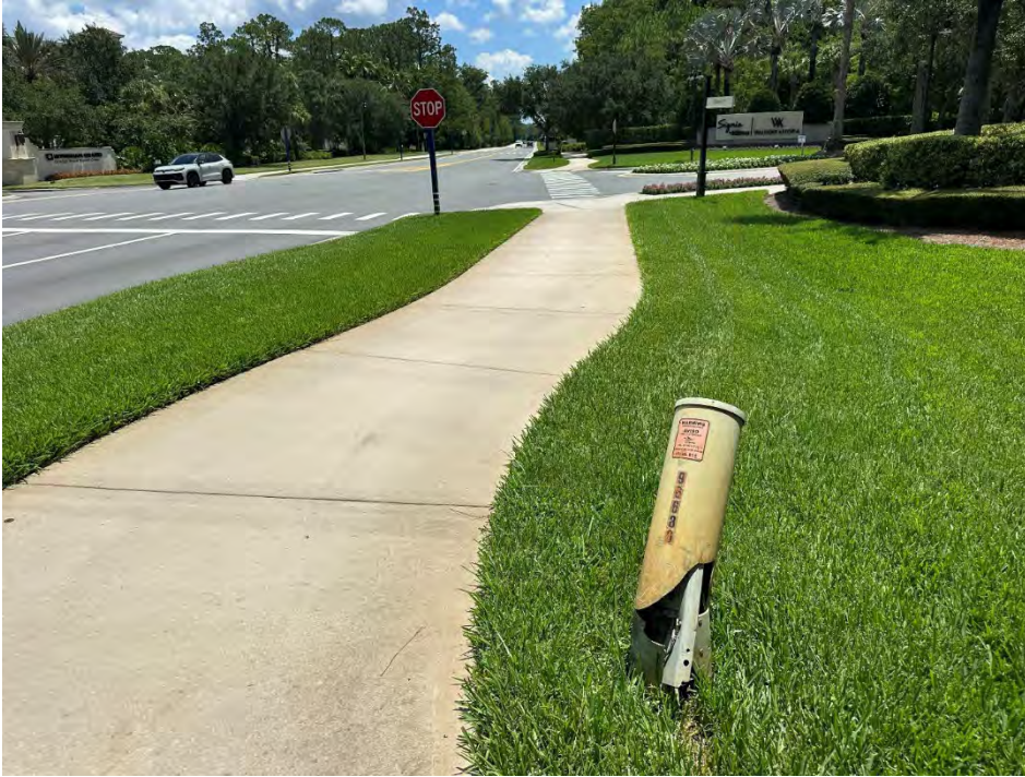
PHOTO 61 Cable covering- broken
