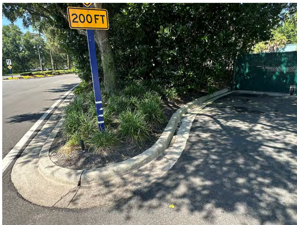
PHOTO 1 Concrete curb- broken/cracking
