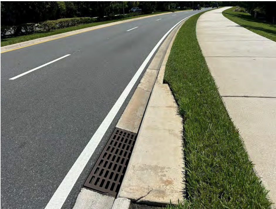
PHOTO 32 Pre-cast Inlet- broken/cracking
