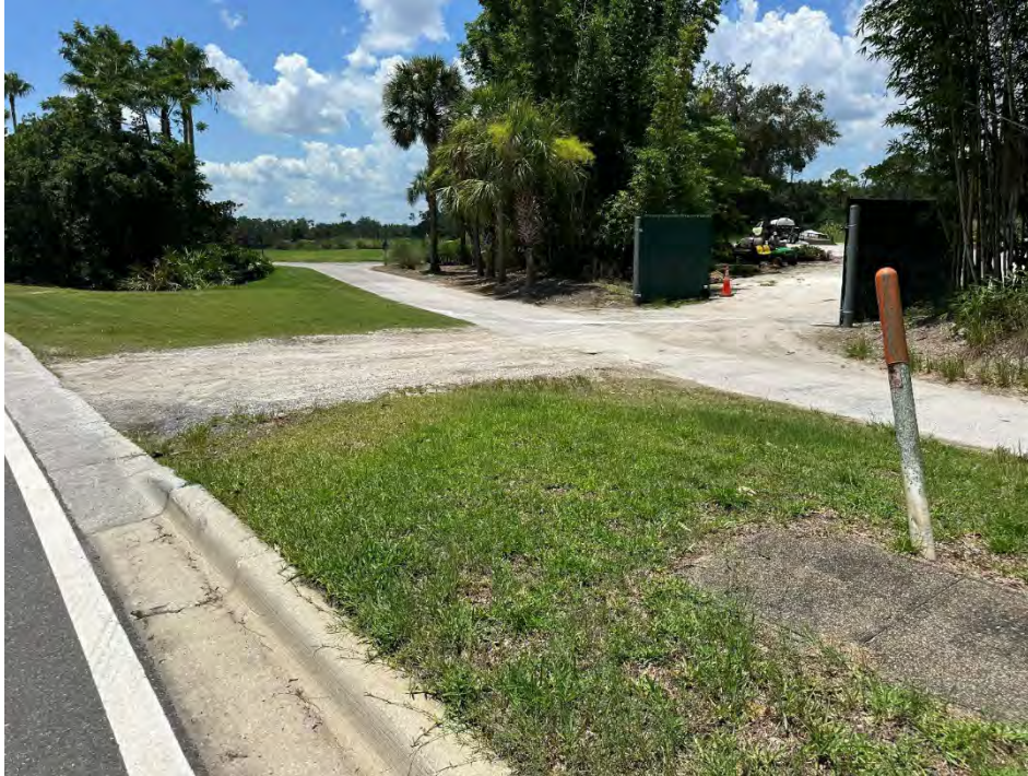
PHOTO 67 Fiberoptic cable marker- over-turned
