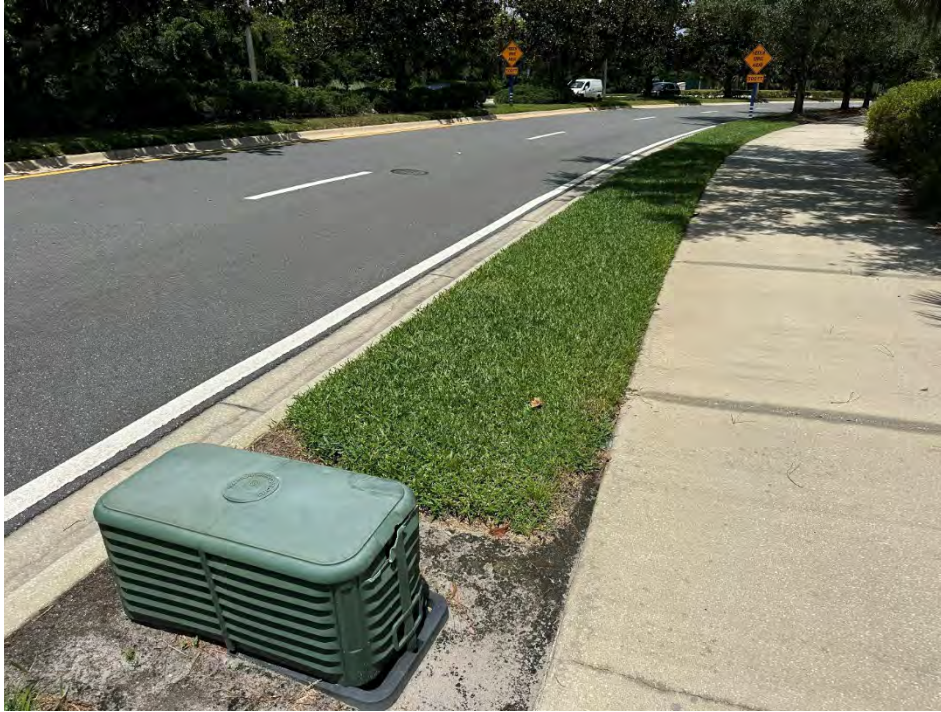
PHOTO 47 Communication box/covering- broken
