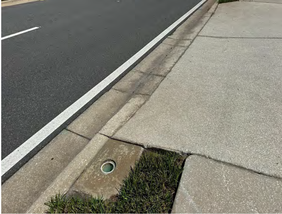
PHOTO 35 Underdrain cleanout- cap broken
