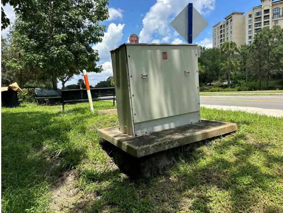
PHOTO 57 Concrete platform- undermined by erosion
