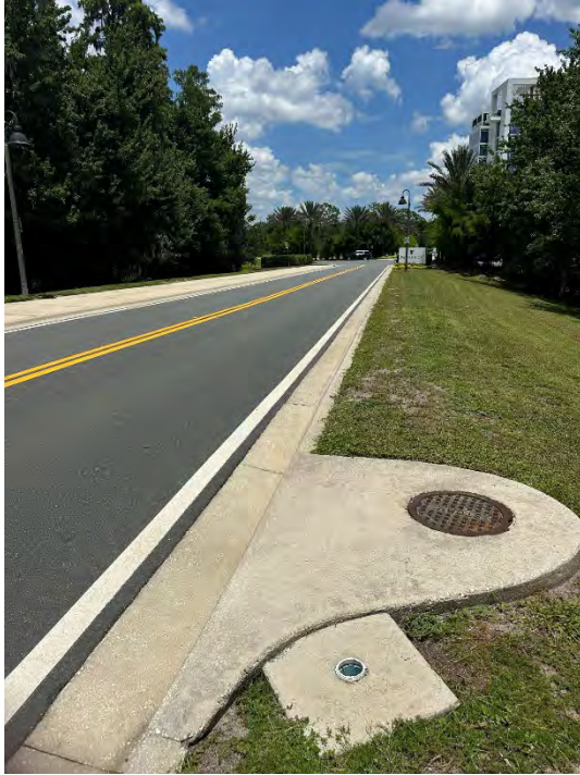
PHOTO 75 Underdrain cleanout- cap broken
