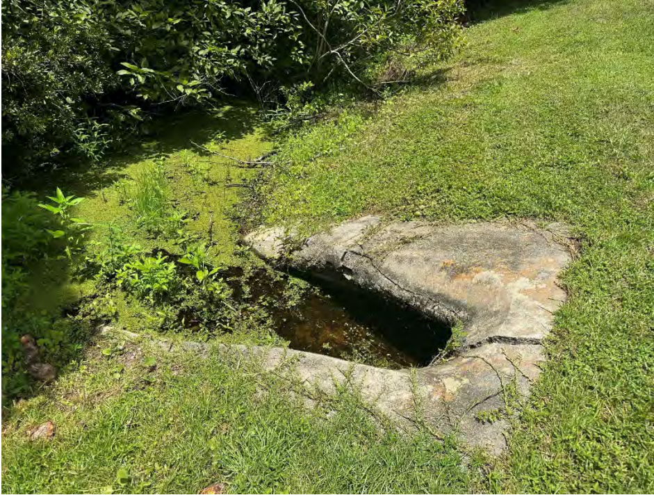
PHOTO 71 Mitered end section- cracks in concrete
