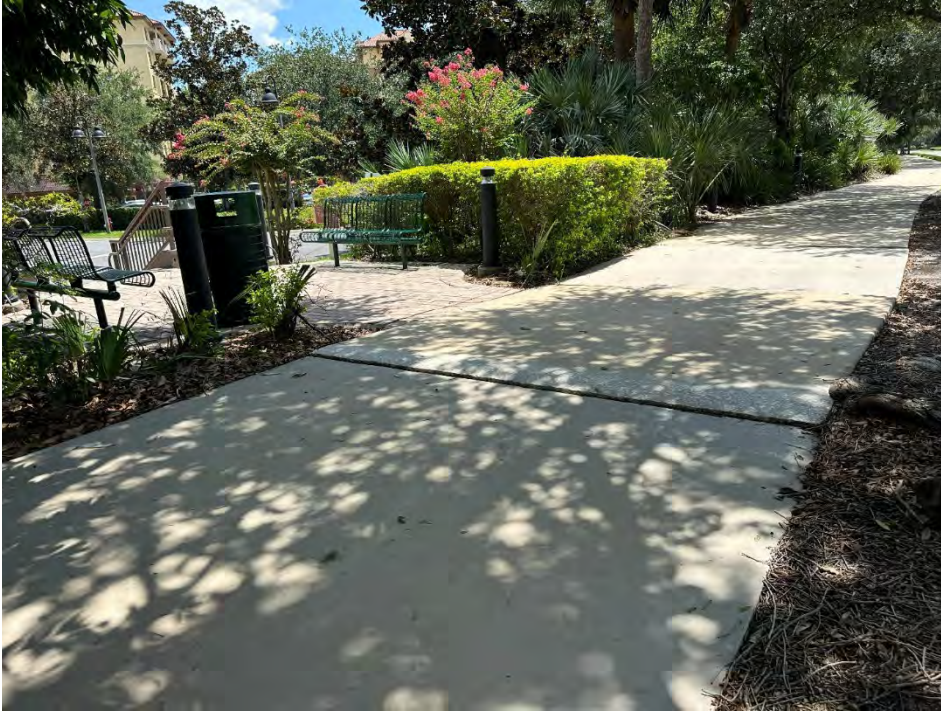
PHOTO 51 Sidewalk- uneven at joints
