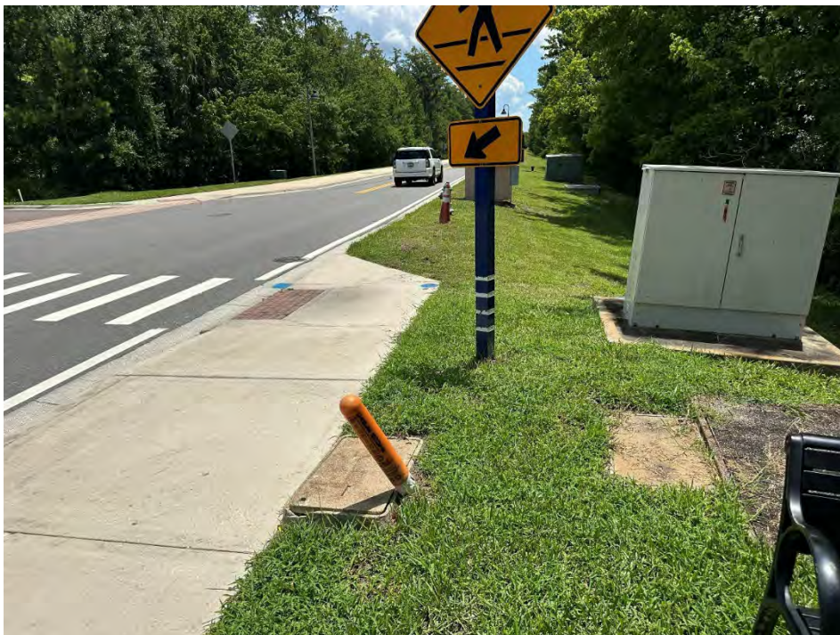
PHOTO 58 Fiberoptic cable marker- over-turned
