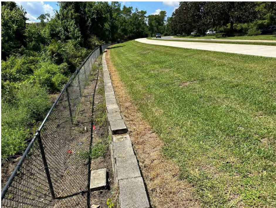
PHOTO 28 Retaining wall- cap blocks displaced
