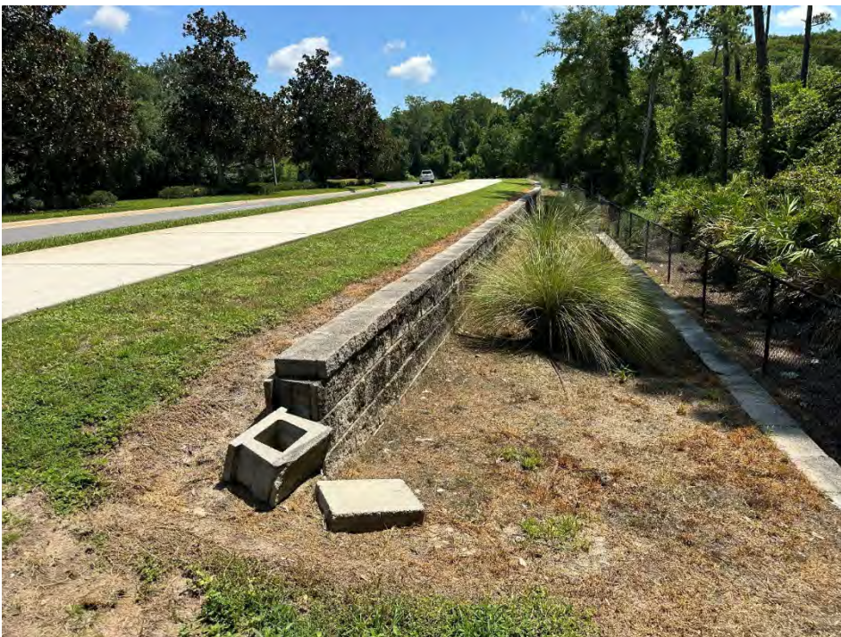
PHOTO 30 Retaining wall- blocks displaced
