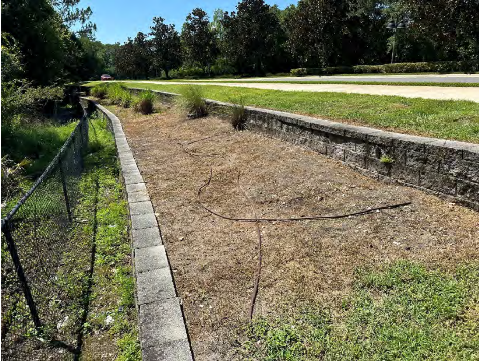
PHOTO 21 Irrigation lines- exposed
