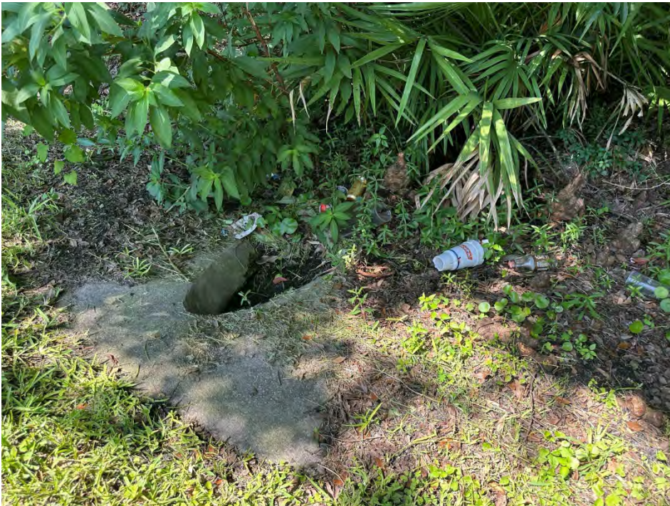
PHOTO 12 Mitered end section- excess debris
