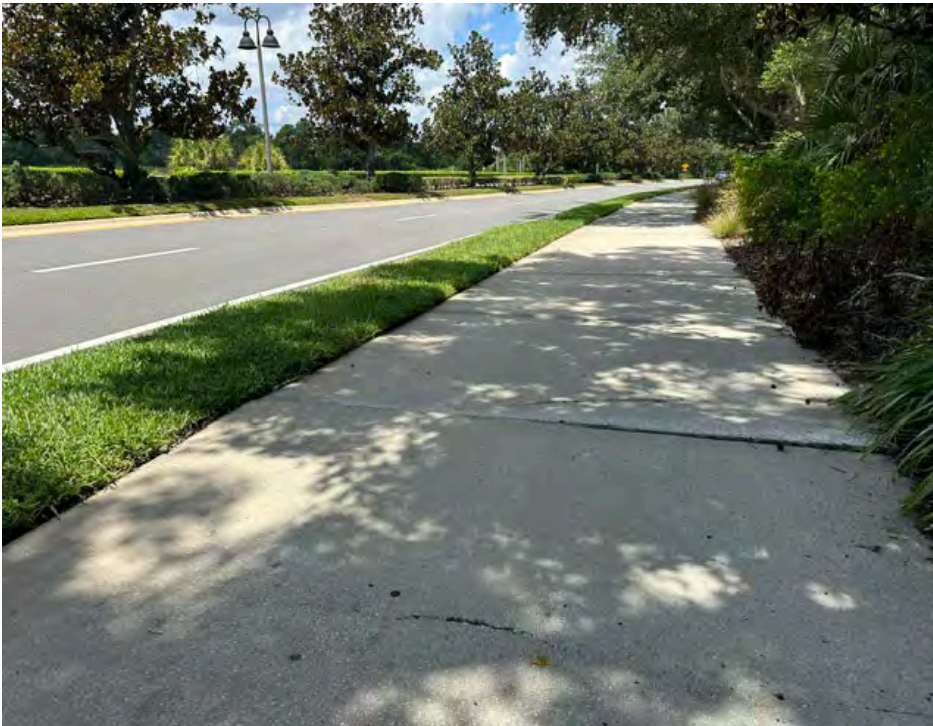
PHOTO 50 Sidewalk- broken/cracking, uneven at joints
