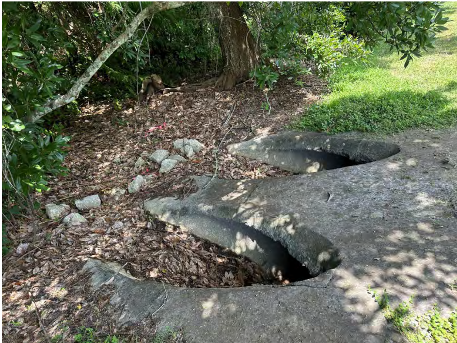
PHOTO 78 Mitered end section- excessive debris impeding flow
