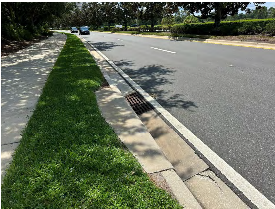
PHOTO 48 Concrete curb- broken/cracking
