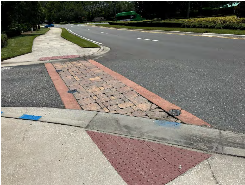
PHOTO 52 ADA ramp/Sidewalk- broken/cracking
