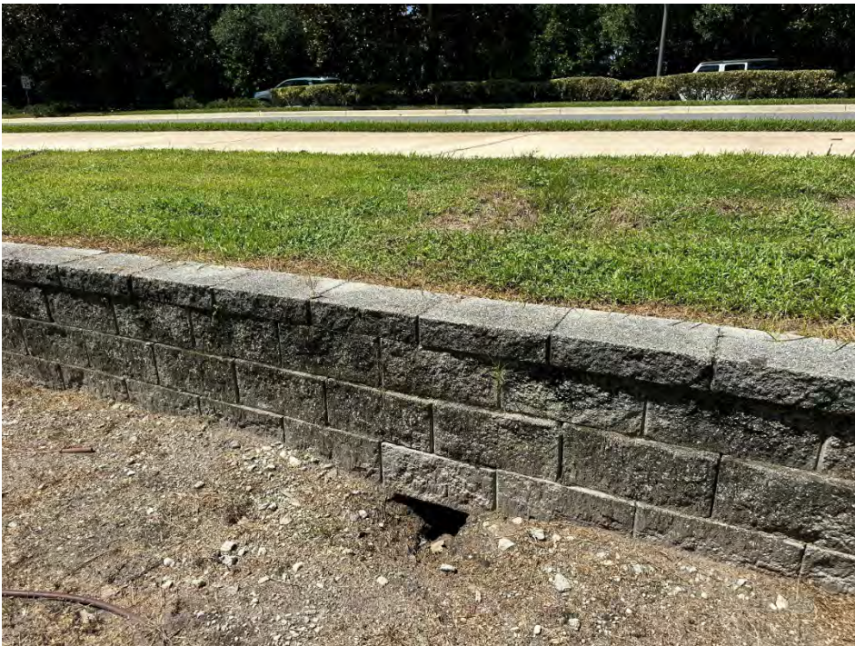
PHOTO 22 Tunneling/burrowing along retaining wall
