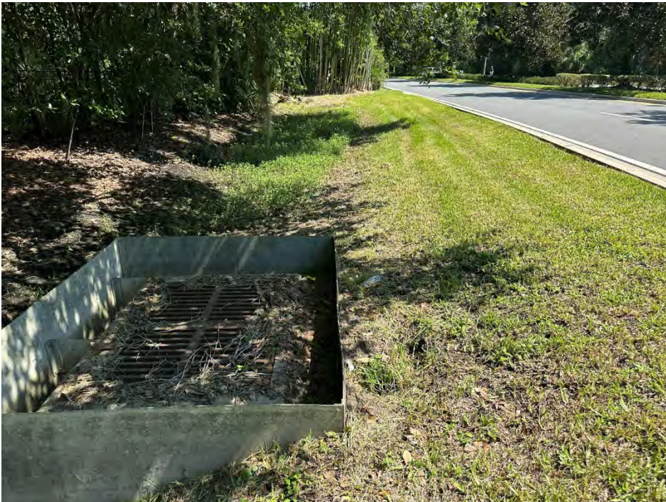
PHOTO 10 Control structure- debris on grate
