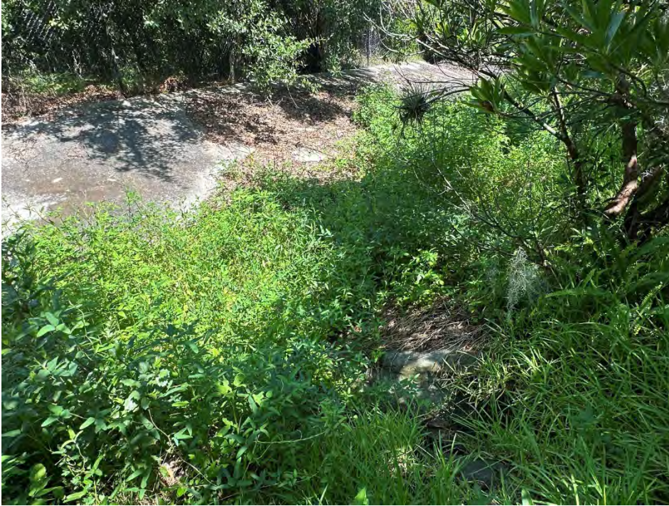
PHOTO 11 Swale- Excess vegetation growth
