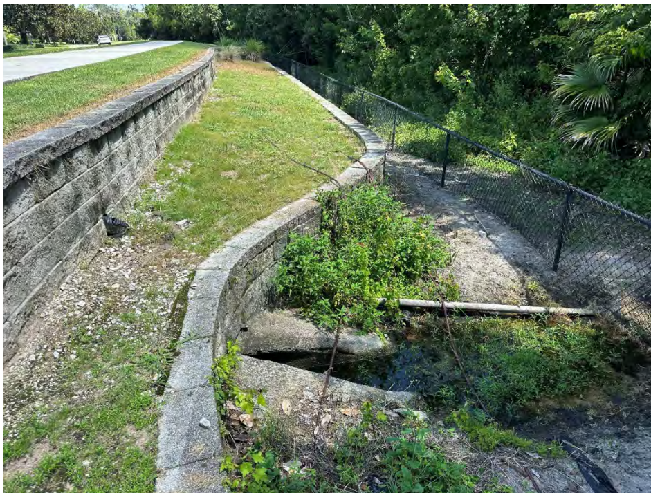
PHOTO 26 Mitered end section- excess debris/vegetation growth, Irrigation lines- exposed
