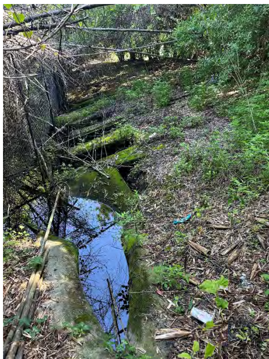
PHOTO 4 Mitered end sections- with ground erosion, cracks in concrete
