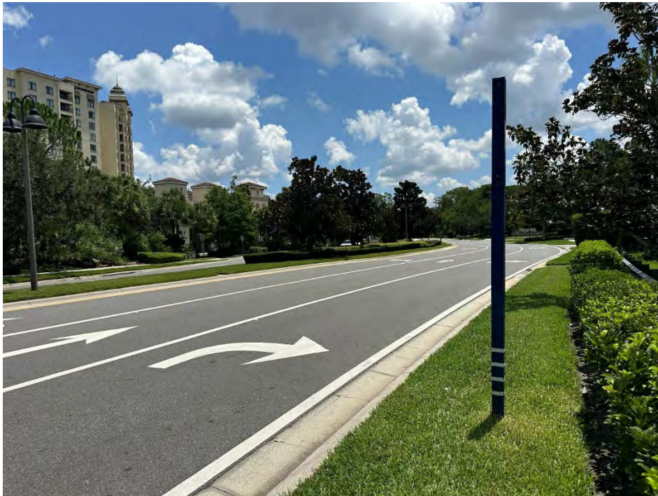
PHOTO 64 Sign panel- missing
