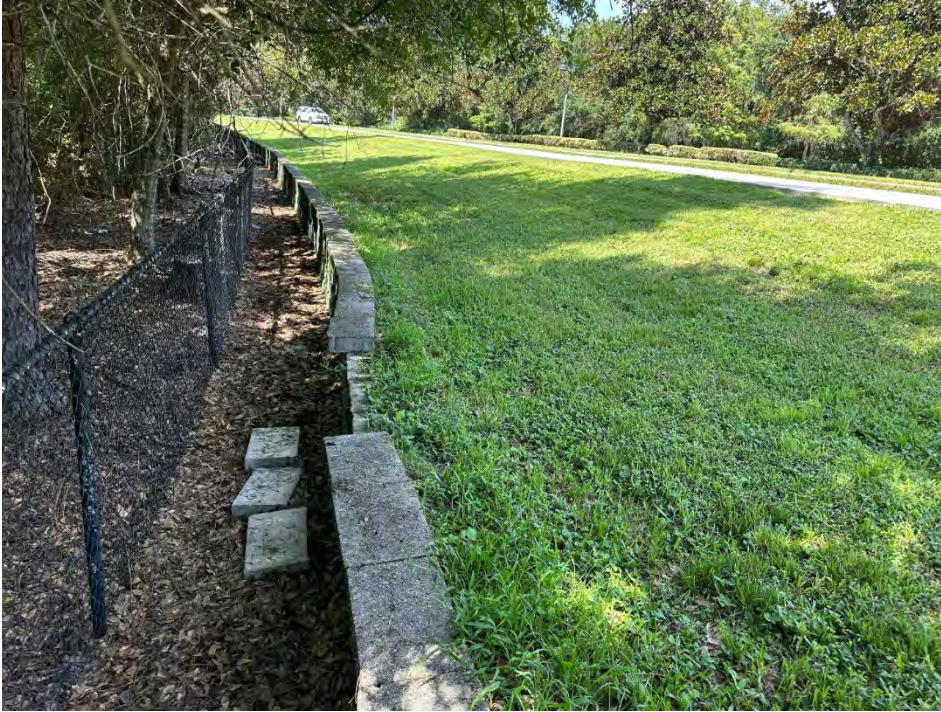
PHOTO 31 Retaining wall- cap blocks displaced
