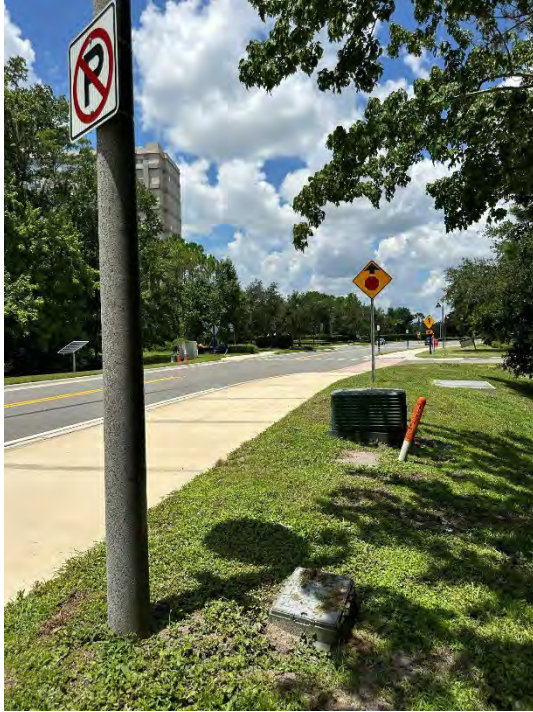
PHOTO 55 Fiberoptic cable marker- over-turned
