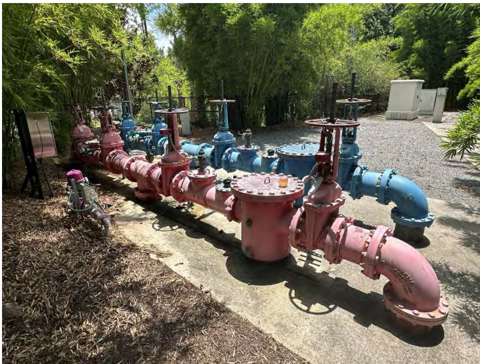
PHOTO 76 Backflow preventer assembly- paint coat fading
